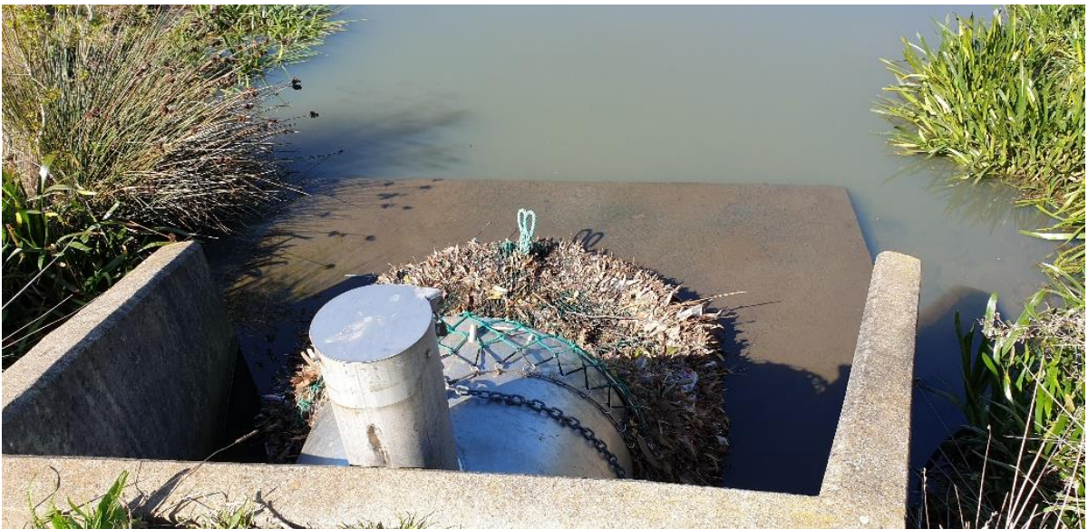
Figure 24. Installed litter net
