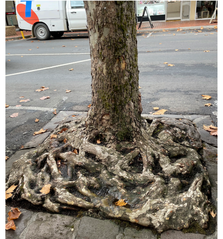
Tree roots protruding more than 30cm above the surface
