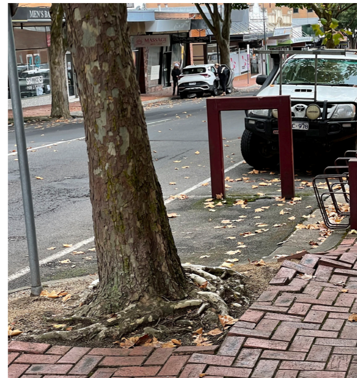
Brick pavers lifted by tree roots
