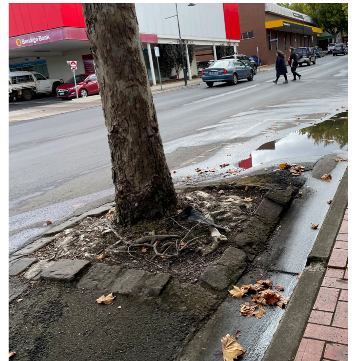
Tree that has lifted the road surface creating drainage issues
