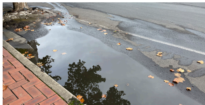
Drainage issues identified on the streetscape
