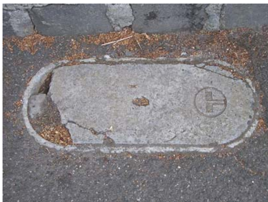
Example: damaged telecoms pit lid in a footpath is a potential hazard to pedestrians. (Photo source ARRB).
